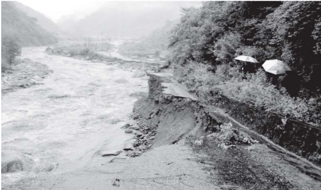
The portion of road washed away by flash flooding in Lungtenzampa, Trashigang in 1994 (DoR)
